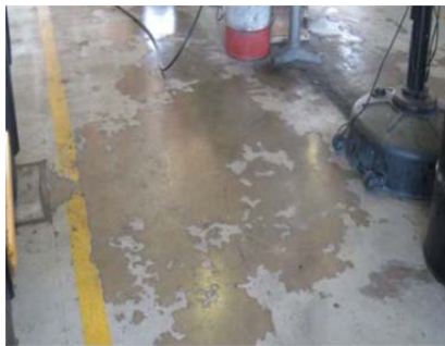
Degrading floor sealant
