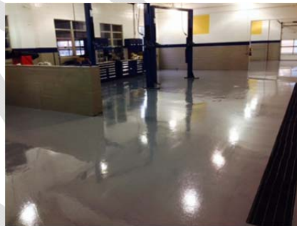
Properly maintained floor sealant
